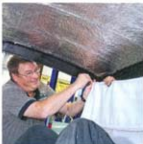
6 Ron Bramlett of Mustangs Plus helps Richard clear the first hurdle of headliner installation, which begins at the rear with the first bow. Some prefer to begin in front. However, if you're going to have problems, it's better if they're in the rear. Each bow location yields at least two pairs of attachment holes to give you flexibility because no two headliner kits are alike.
