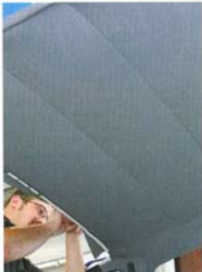
19 Headliner is completely secured front and rear. There are a few minor wrinkles to be ironed out with a heat gun or hair dryer.
